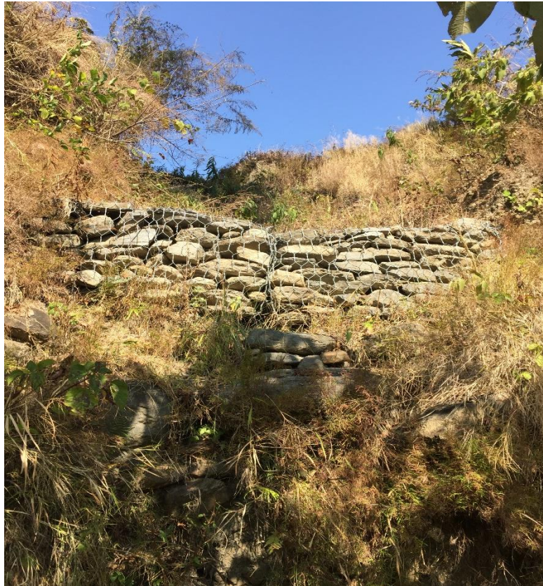
Photograph 11: Gabion wall as control measure of landslide
