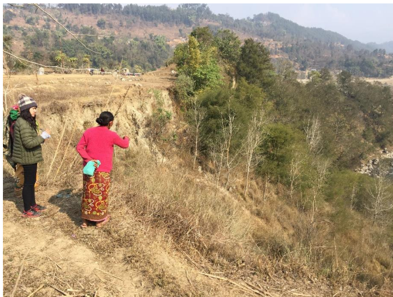
Photograph 12: Landslide caused due to the river cut-off
