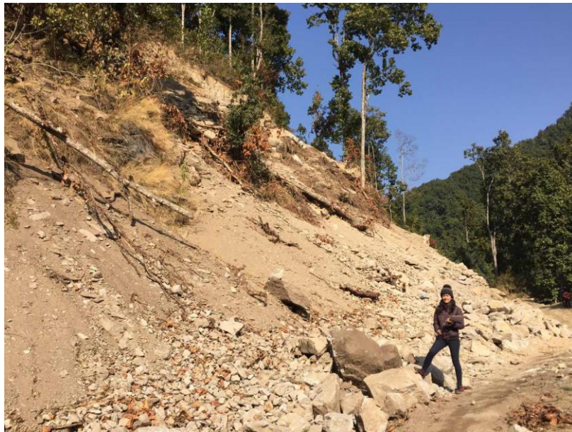
Photograph 4: Landslide in the study area
