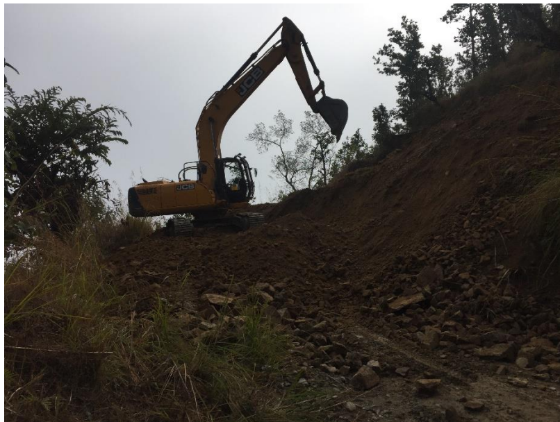
Photograph 10: Unmanaged road construction causing downfall of the slope area
